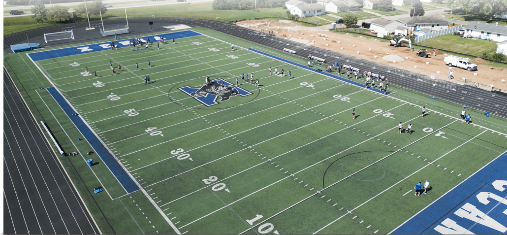
A view of Doug Adams Stadium in July 2023, the old stands demolished and the groundwork being laid for the new grandstands, LED lights, and premium sound.
